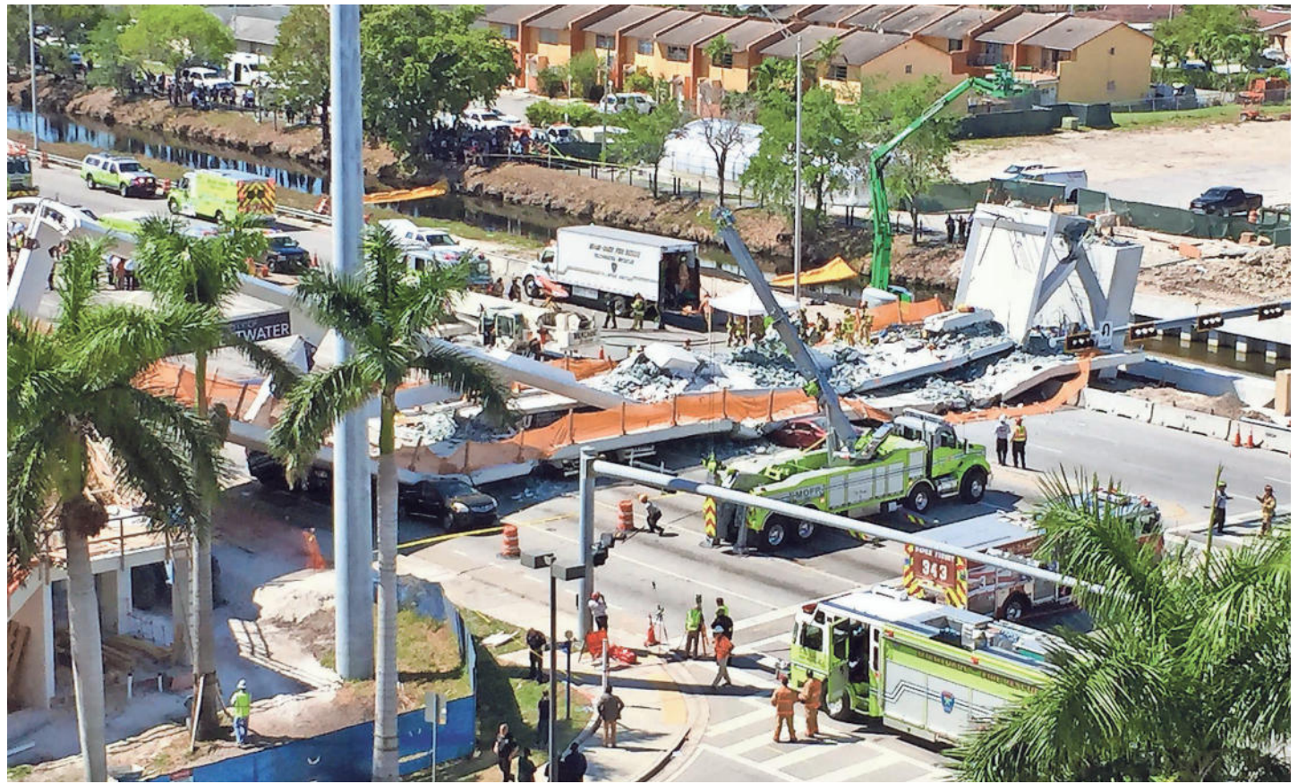
Emergency workers respond to a collapsed pedestrian bridge at Florida International University on Thursday in the Miami area. Search-and-rescue teams used dogs and cranes to go through the rubble. ALAN GOMEZ/USA TODAY
